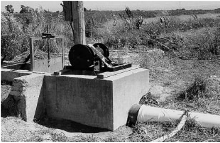
Concrete head ditch with siphon tubes.
