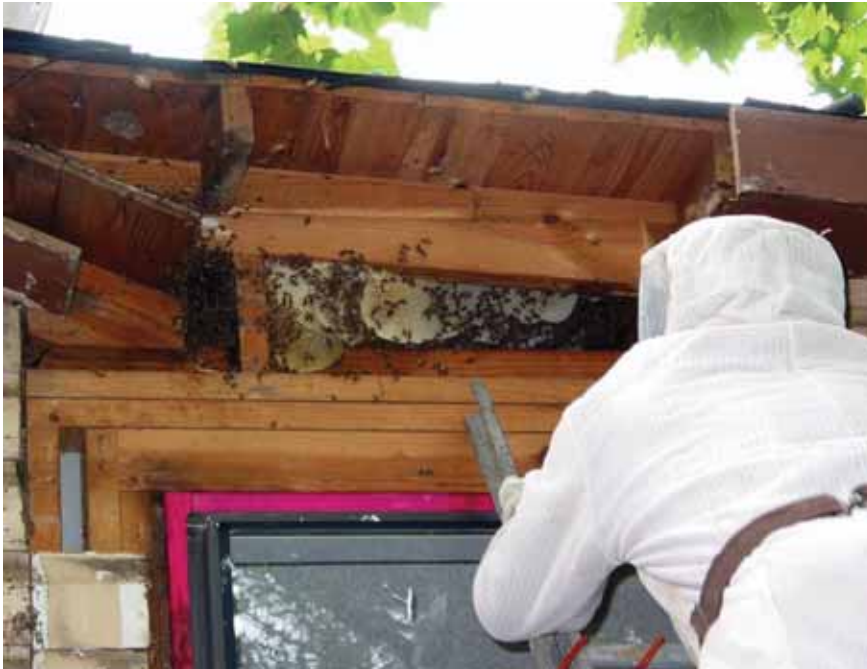
Figure 4. Honey bee nest and worker bees are exposed within a home wall void. Nest removal from buildings is a job for professional pest control services. Photo by Timothy Haley, USDA Forest Service, www.insectimages.org
